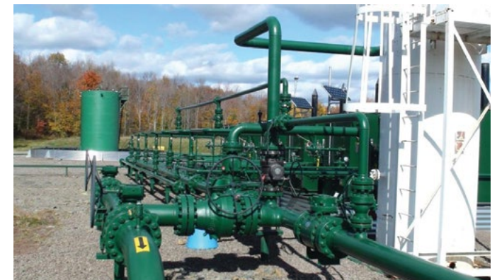
Natural Gas Production Header
