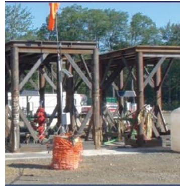
Well Head Cages for Infield Drilling
